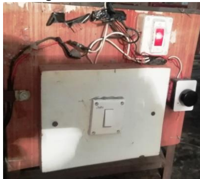
Figure.3 Control panel of air heater
