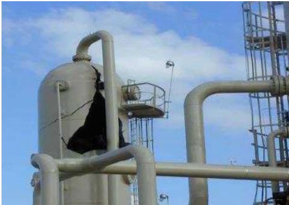
Fig. 2. Failure of pressure vessel during hydro Test.
