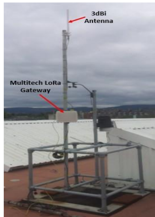
Fig. 2. LoRaWan Gateway installation
