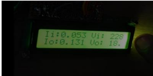
Monitoring of voltage and current (primary and secondary)
