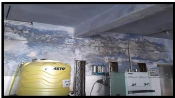
Figure 6: Seepage in wall
