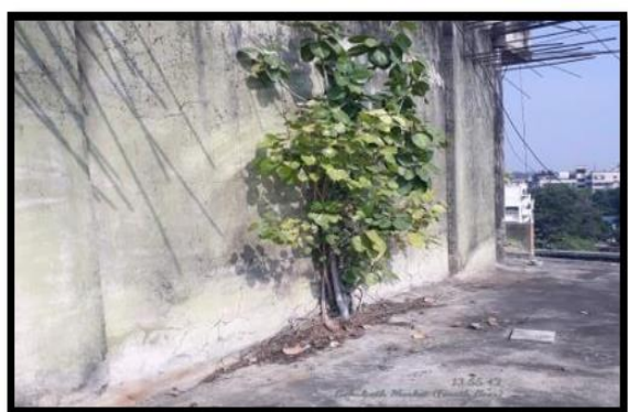
Figure 7: Vegetation Growth on structure
