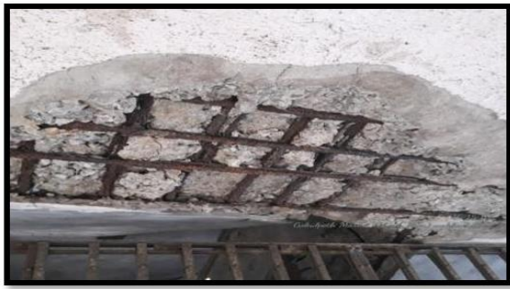
Figure 5: Reinforcement exposed and concrete damage
