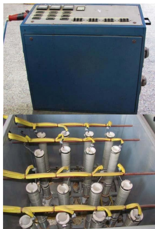
Fig. 1. Three-phase and single-phase resistors.
